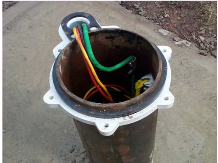
FIGURE 15-13: ELECTRICAL WIRES - CLOSE UP
