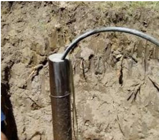
FIGURE 15-34: PLUGGING MATERIAL COMING OUT OF CASING
