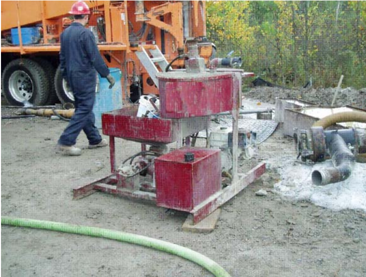
FIGURE 15-29: GROUT MIXING MACHINE
