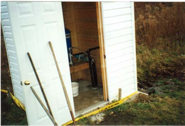
FIGURE 15-11: DRILLED WELL INSIDE A PUMP HOUSE
