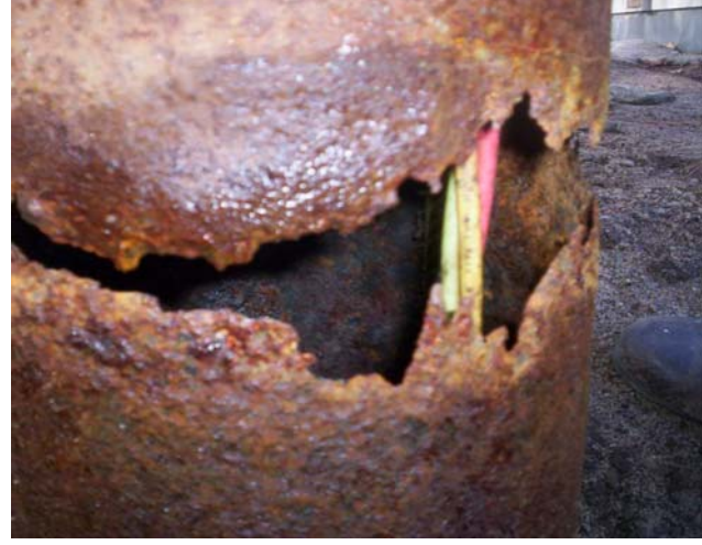
FIGURE 15-21: CORRODED CASING FROM OUTSIDE
