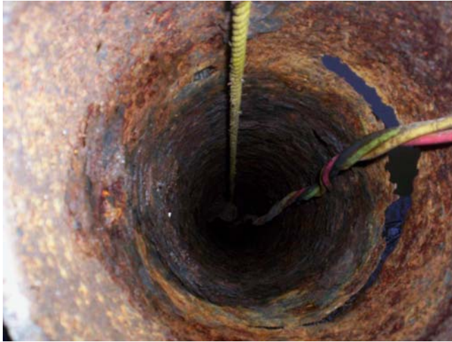
FIGURE 15-20: CORRODED CASING FROM INSIDE
