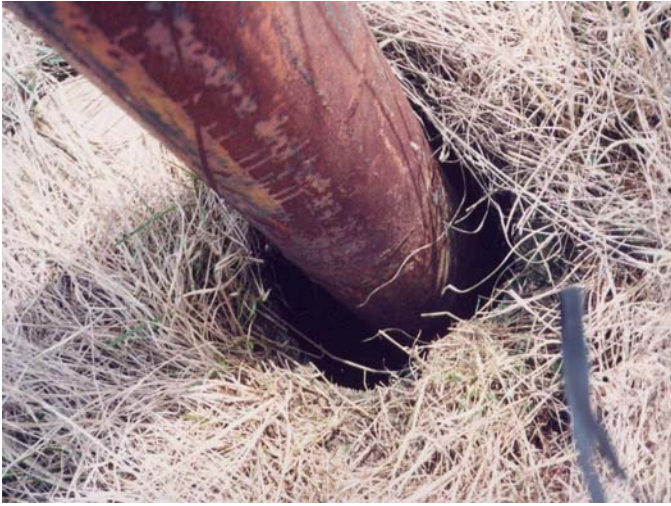
FIGURE 6-3: VISIBLE OPEN ANNULAR SPACE ADJACENT TO DRILLED WELL CASING
