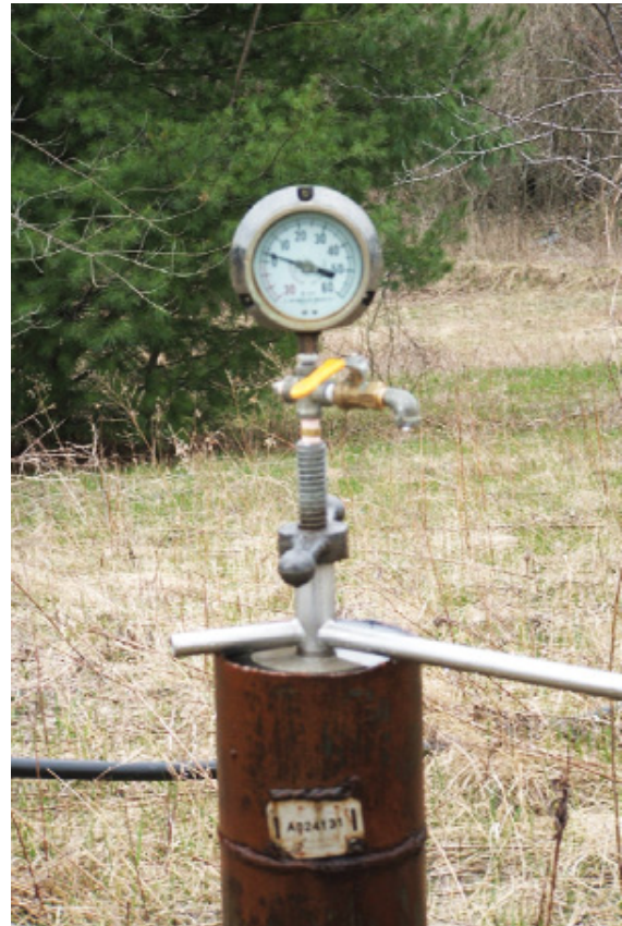
FIGURE 12-5: FLOWING WELL PRESSURE GAUGE DEVICE - INSTALLED
